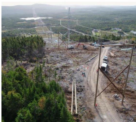
Figure 5: Wooden Pole Solution Used in 2018 Mock Exercise
