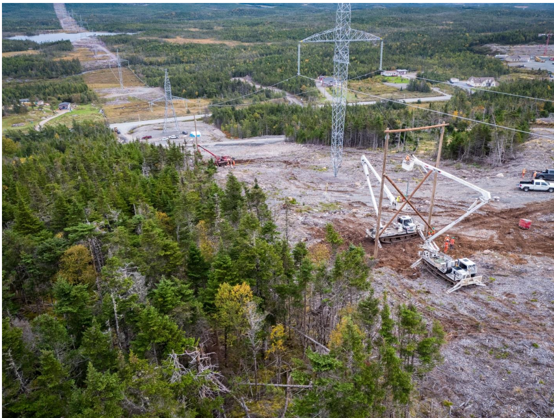
Figure 6 - View Down the Line
